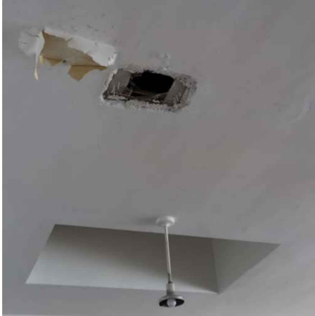
Emergency Operations Center
